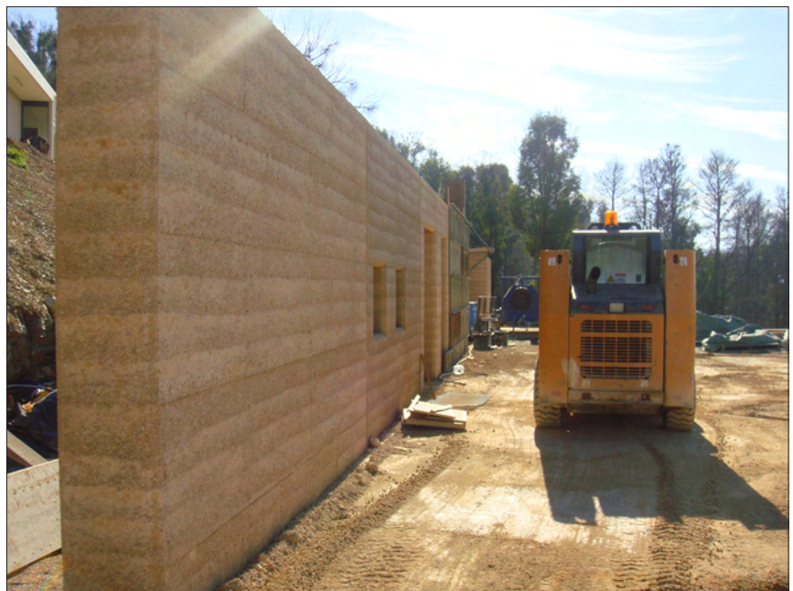
Top: The versatile grid-connect PV system can also operate independently thanks to a battery backup. Bottom: Beautiful and fire-resistant rammed earth walls on the western and northern sides during construction.
